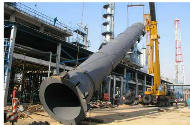
汽提塔 Stripping tower
